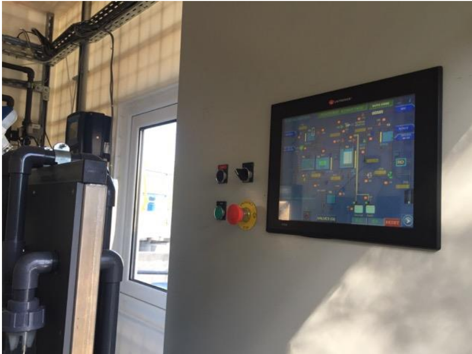
Figure 14: PLC HMI Installation at KEREFT Pilot Site
